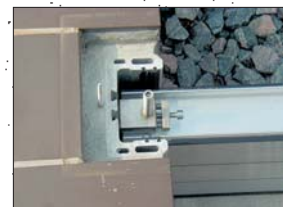
In the recessed cut-out
