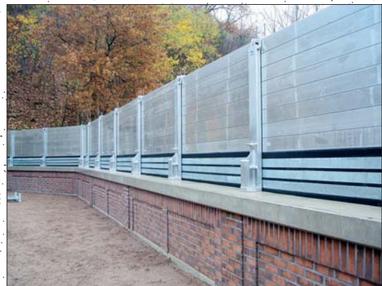
Hot galvanized steel dam beams up to HQ 100 level
