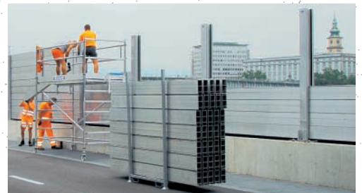
In two construction stages a barrier height of 2.50 m is reached with only ten dam beams per section
